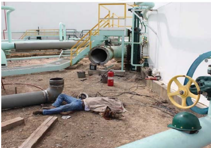
Figure 1: A welder with more than 20 years' experience, was killed in an explosion at a crude oil storage facility in the ship channel in 2012.
