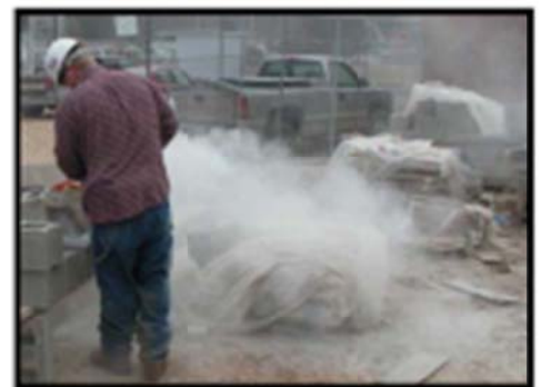
Concrete cutting with saw creates obvious dust exposure.
